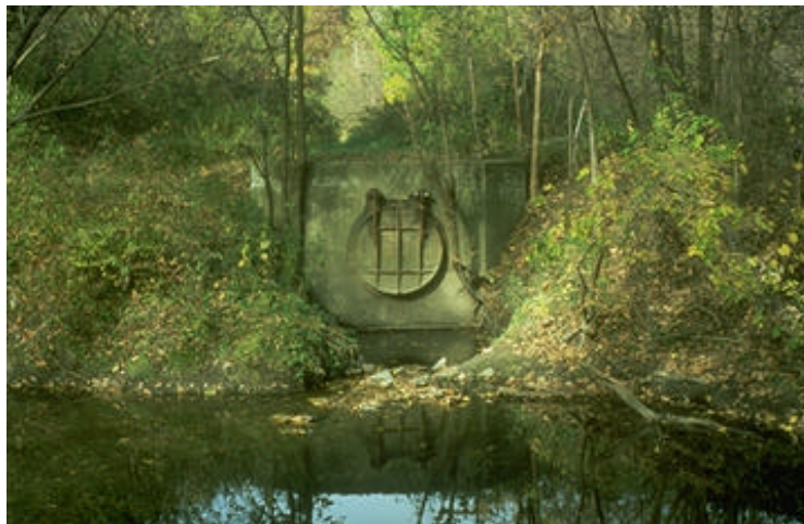
A. Uncontrolled CSO Discharge on the Rouge River
