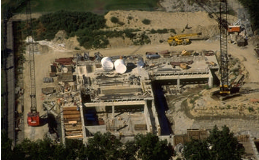
B. Redford Township CSO Retention and treatment basin on Upper Rouge River Under construction (1994–1996)
